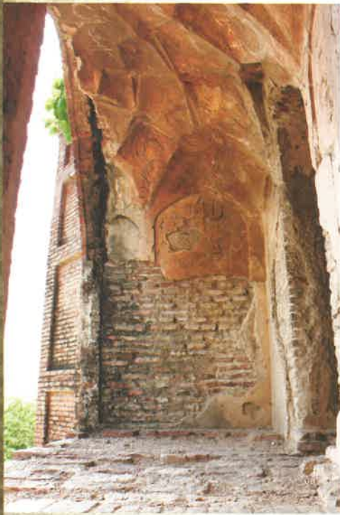
Damaged portion of the Stalactite at the upper portion of the tomb.
