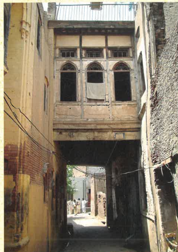
Bhera – Heritage of this once a glorious town is crumbling rapidly.
