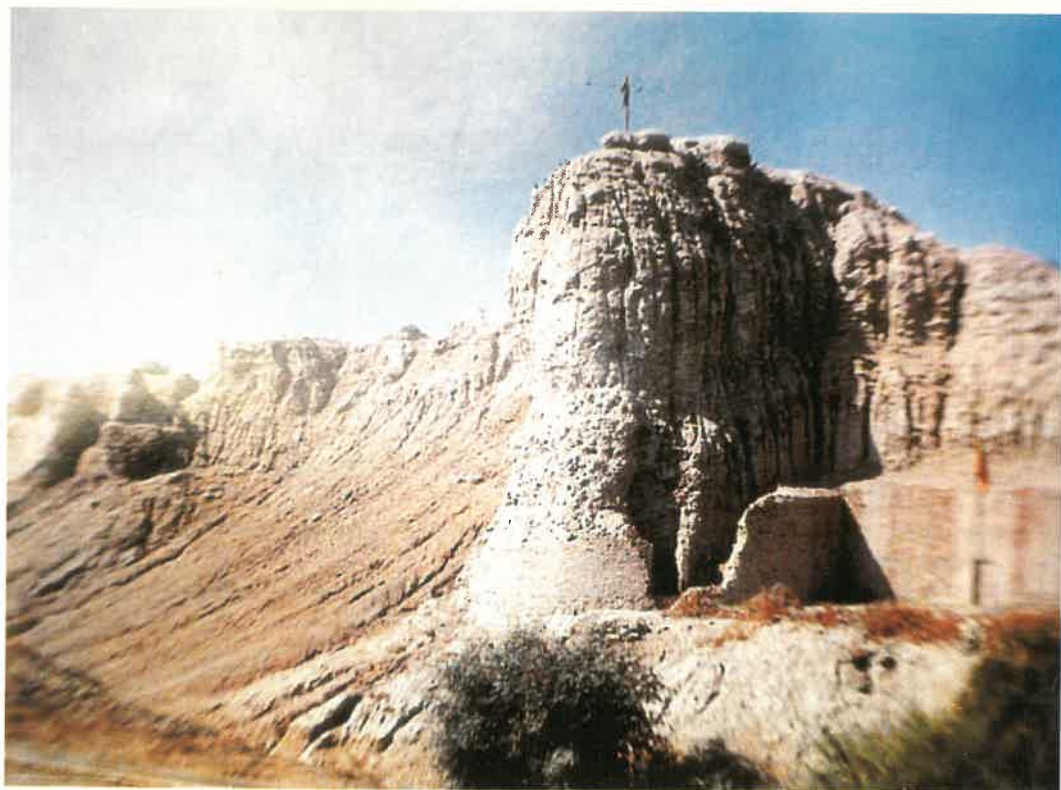
Shwan Fort: General View of decayed fortification and bastion
