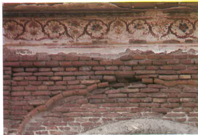
Peeling plaster and paint on the facade of Shish Mahal.
