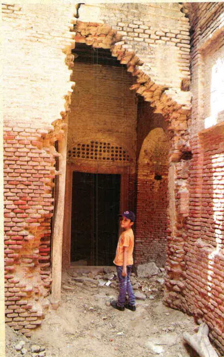
Decay in progress.
