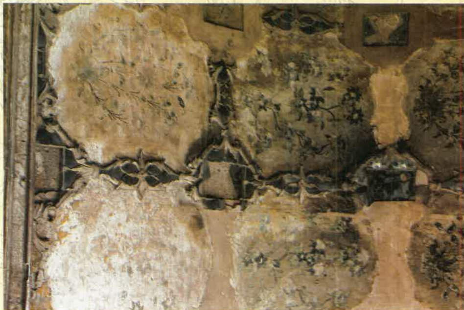
A deteriorated artwork in Shish Mahal.
