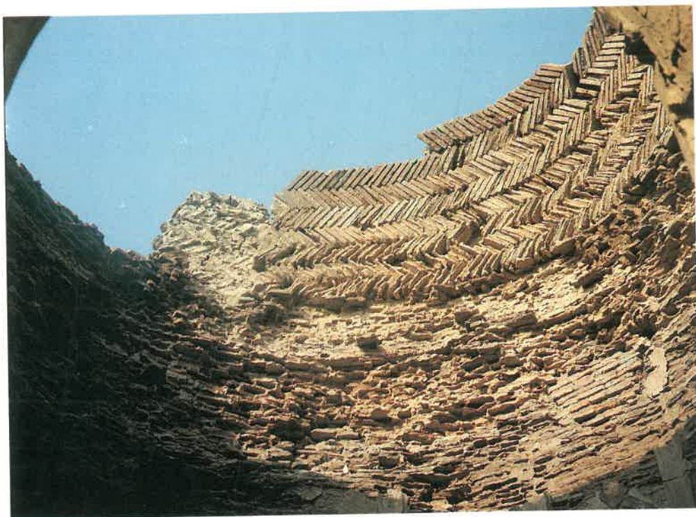
Tomb of Hamsheera (sister) Fateh Khan - Interior view of collapsed dome.
