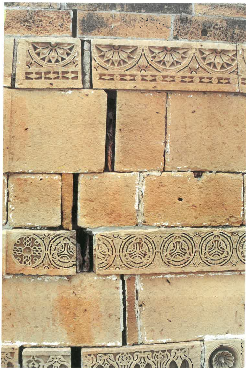
Open joints of stone masonry exposed to hazards (Photo courtesy Asef Nadiem).
