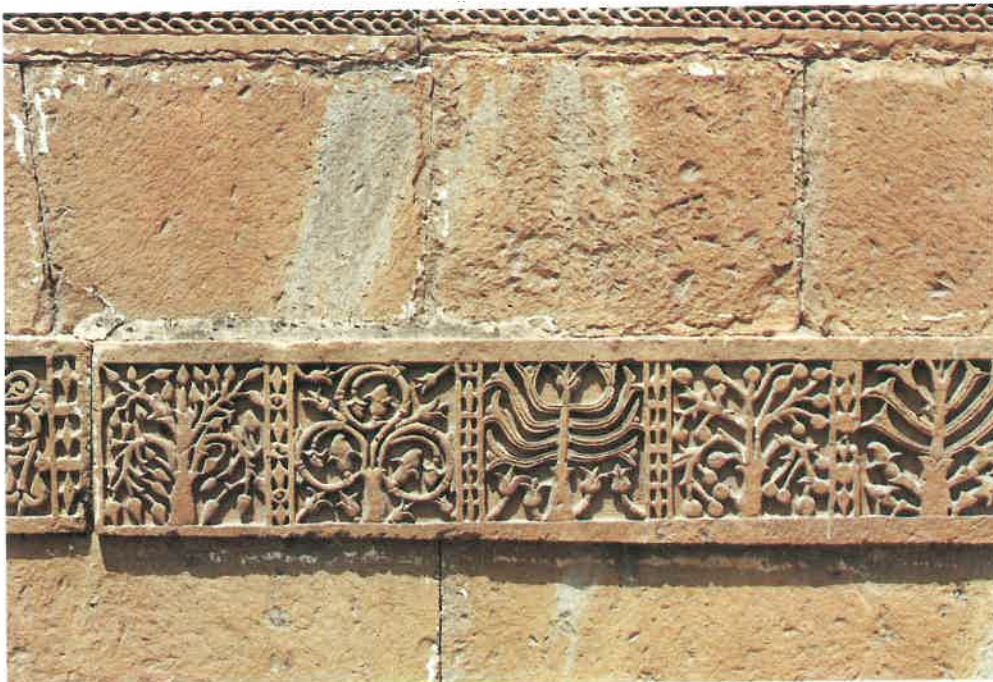
Stone surface roughened due to exposure to direct rain. (Photo courtesy Asef Nadiem).
