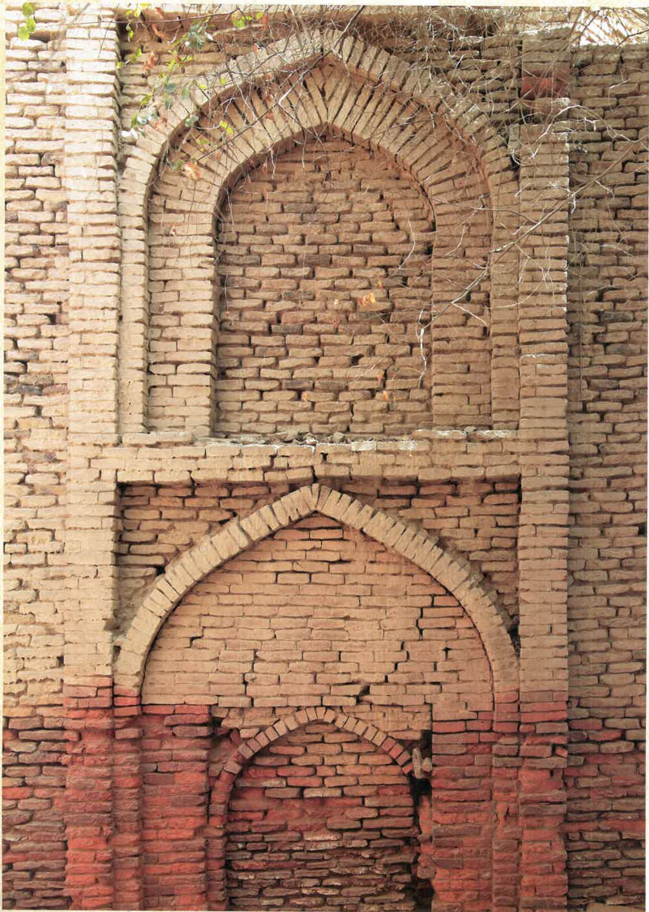
Detail showing deteriorating condition of the structure.
