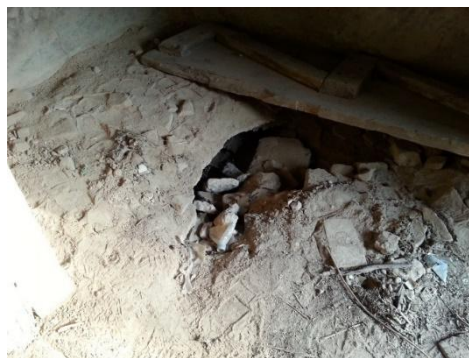
Figure 5-20: Image showing damage floors
