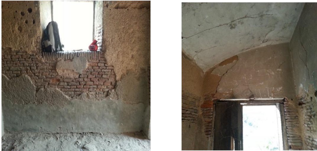
Figure 5-17: Damaged Plaster, Cracks in Building, Damaged Brick Masonry, and Decayed Wood
