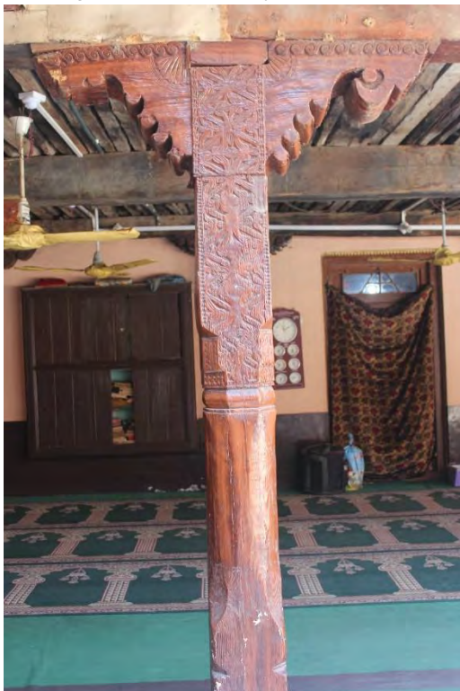
Fig. 32. Wooden capital and pillar at Loye Jumaat (big mosque), Khwazakhela, Swat.
