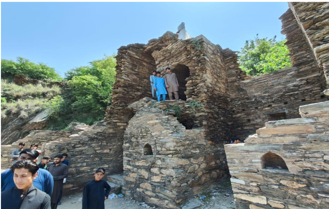
Pl 2: Visitors are climbing the walls of the Takht-i-Bahi Monastery causing the serious damages
